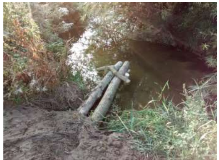
Flow deflector keyed into bank and held in place with posts driven into the channel bed.
