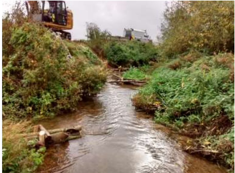
Looking downstream at a series of flow defectors to create channel sinuosity.
