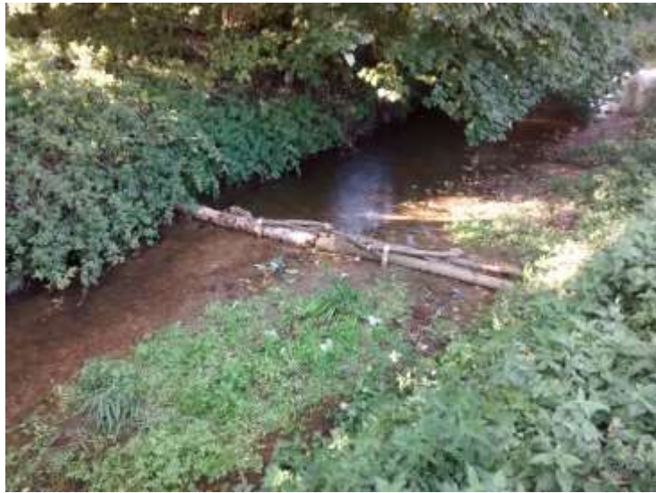
Log jam across full channel width, to create bed scour immediately downstream.
